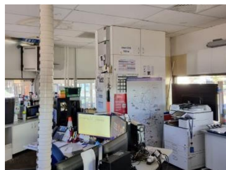
Figure 28 – crowded interior of Operations Room. Note water leak in ceiling
