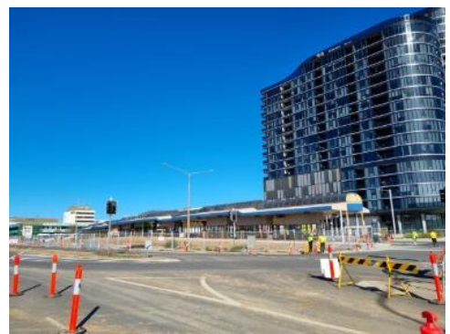
Figure 16 – View south on Callam Street. Note the dominance of tower to right
