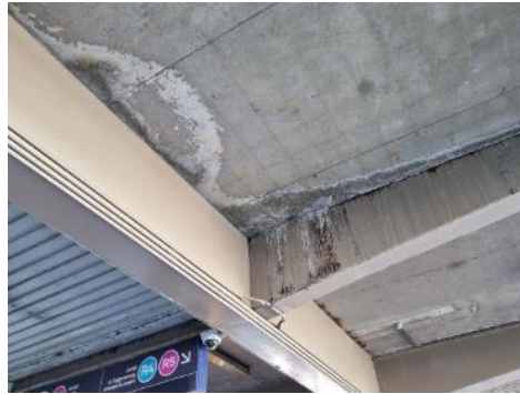
Figure 32 – Water Leaks in stage 1 canopy
