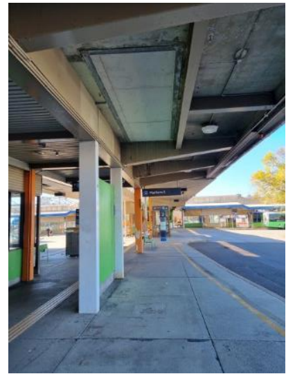
Figure 19 – Typical original canopy structure. Note location of stair in soffit and pavement changes
