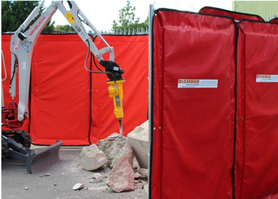
Figure 3.12 Example of a temporary noise barrier
