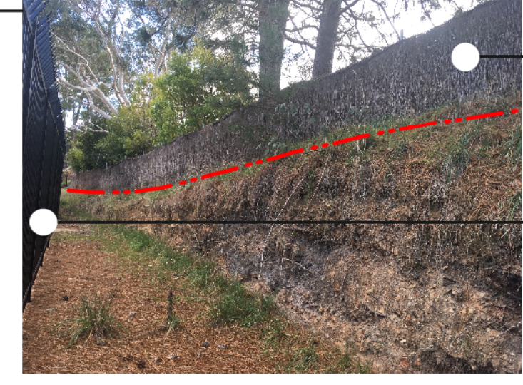
Existing private thatched fence to be retained Boundary Line Existing steel fence to be removed
