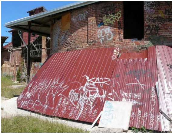
Figure 2.44 Hoffman kiln at the former Standard Brickworks, 2010. (Source: Lovell Chen, 2010, Canberra Brickworks CMP, p 190)
