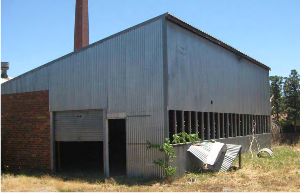
Figure 157 Exterior, showing the south and east elevations. The brick wall is an earlier element incorporated into the workshop building.
