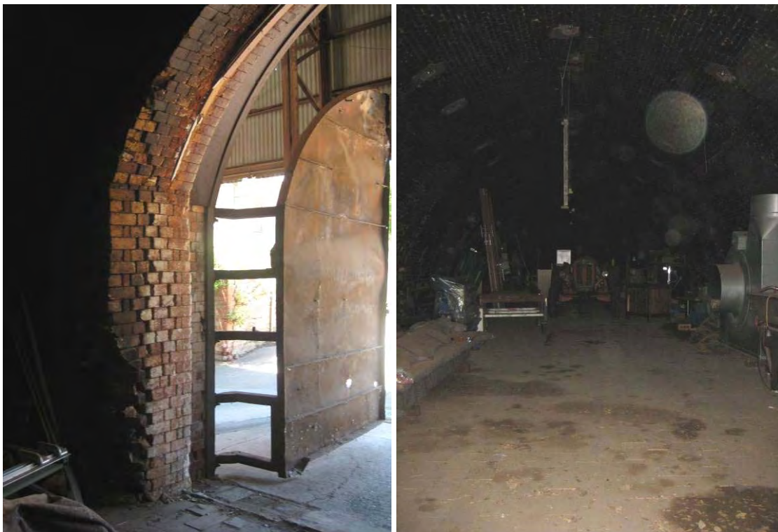
Figure 139 From left: interior of kiln showing entry and deteriorating fire bricks; interior of kiln showing later cement paving.
