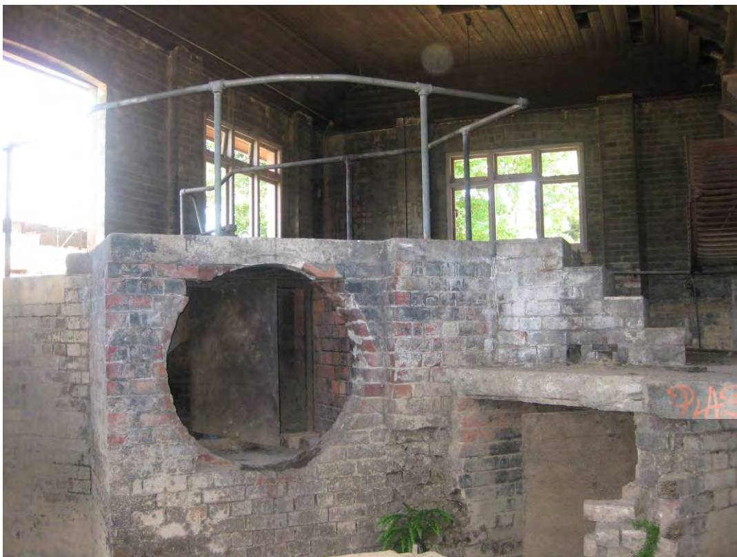
Figure 59 Another view showing the entry to the tunnel / flue connecting the fan house with the Staffordshire kiln.
