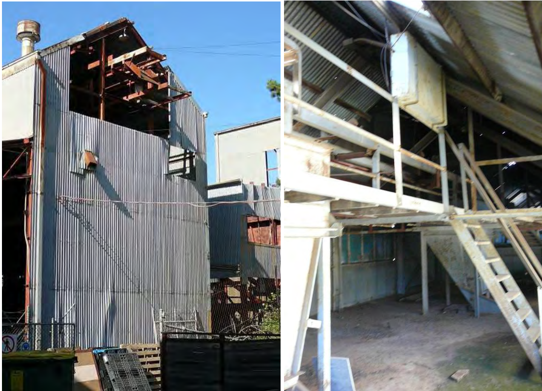
Figure 107 From left: the truncated south end of Machine Bay 1, showing location of former headgear housing; interior of the loft space.
