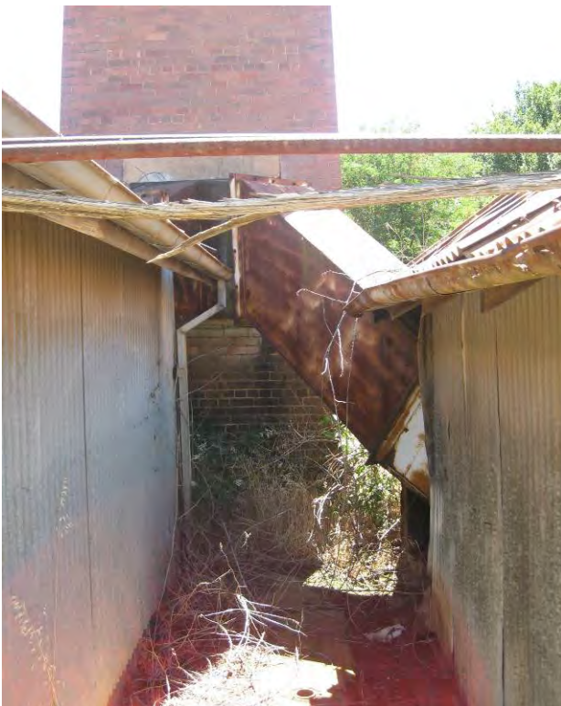
Figure 91 Ducts connect through to the chimney stack.
