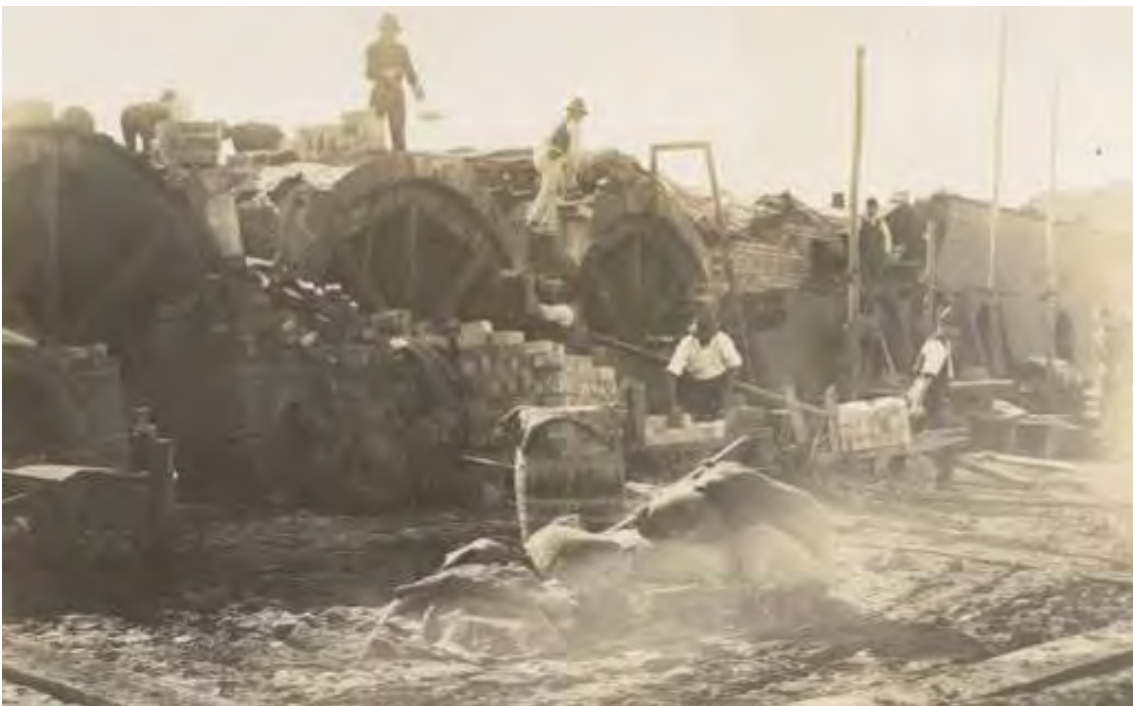
Figure 32 Constructing the transverse arches of the Staffordshire kiln, c. 1915. Source: National Library of Australia.
