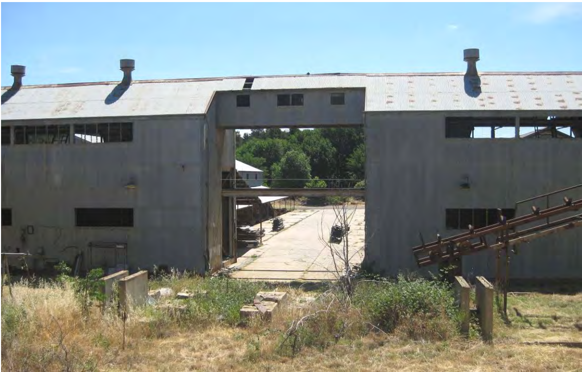
Figure 116 Machine Bays II (left) and III (right), looking west, showing the conveyor 'bridge' and open walkway between the two structures.
