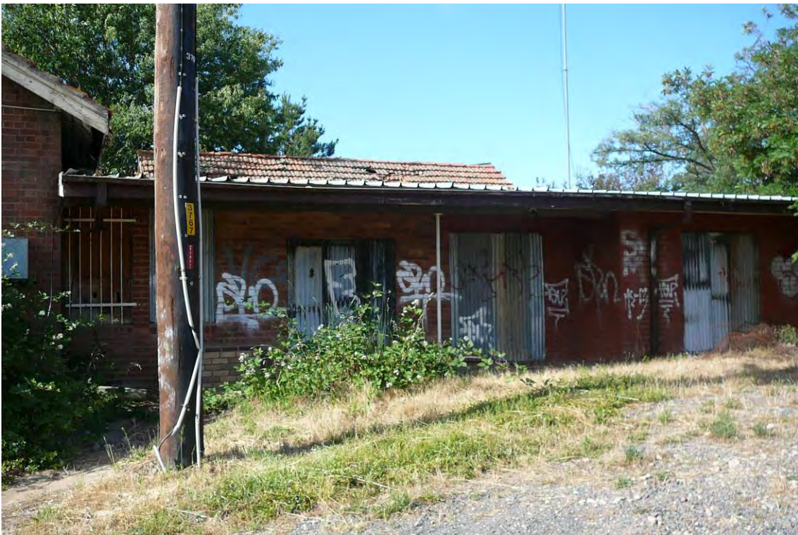
Figure 80 South elevation. Part of the Power House (Building 3) is visible at left.
