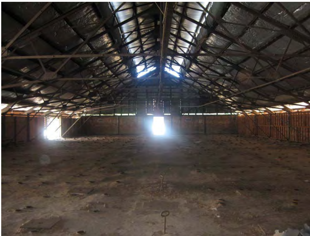
Figure 22 Interior of the firing floor to one of the Hardy patent kilns at the Canberra Brickworks
