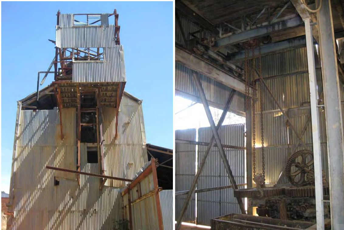
Figure 117 From left: north end Machine Bay III showing remains of headgear housing for the loft conveyor; interior with remnants of the Anderson brick machinery at north end.
