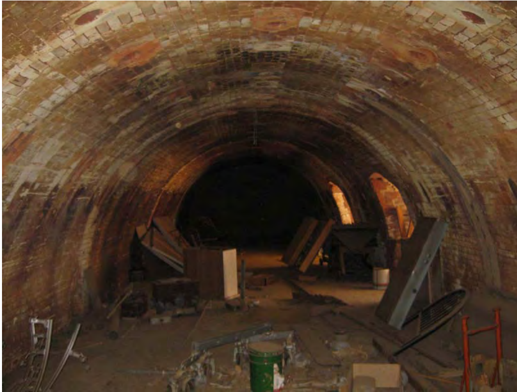
Figure 21 View into the firing chamber of one of the Hardy patent kilns at the Canberra brickworks. Note the wickets (openings) on the right from which the bricks were loaded and unloaded, and the firing holes in the ceiling/walls.
