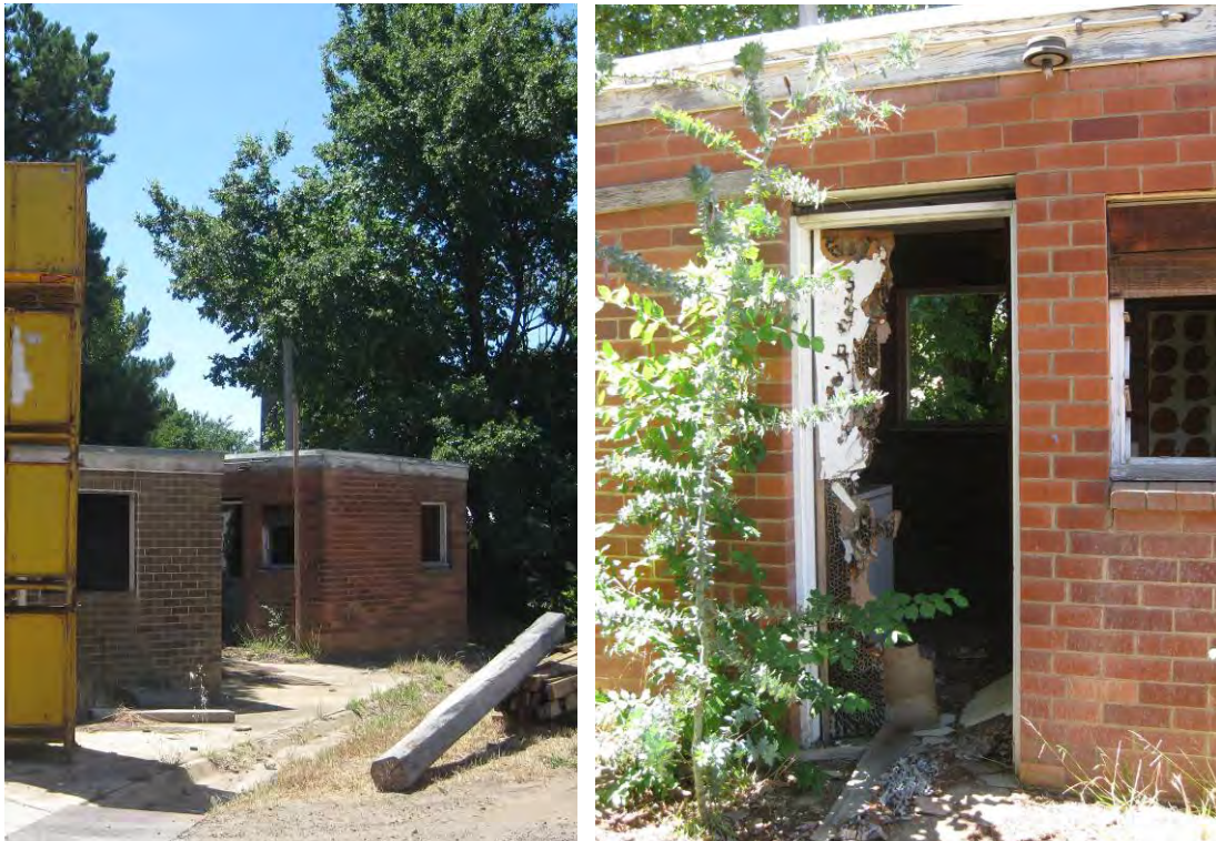
Figure 143 From left: the amenities block is the small red brick building at right; entry.
