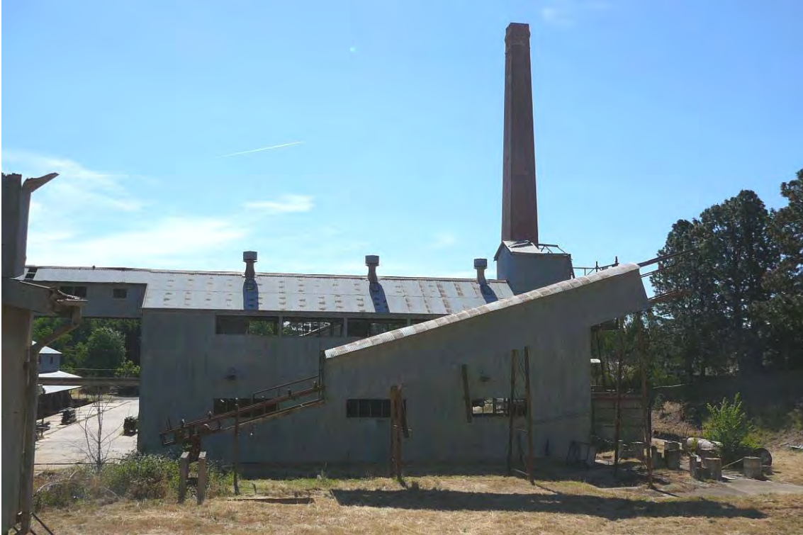
Figure 115 Machine Bay III, east elevation, with the remains of the conveyor in the foreground.
