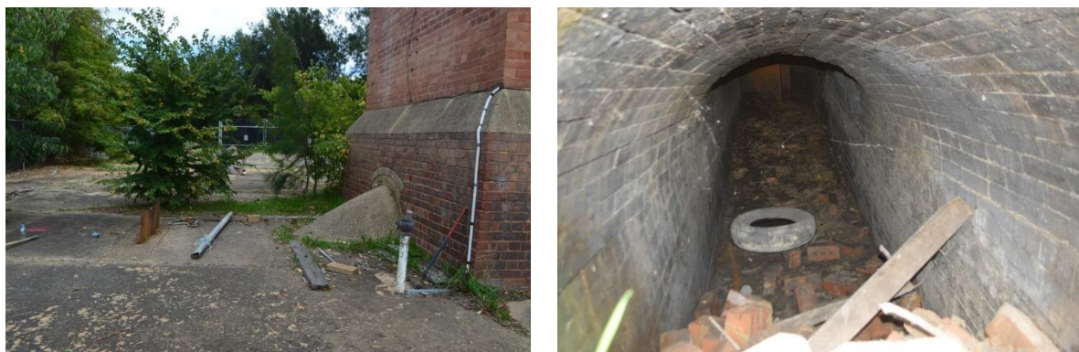
Figure 4.131 Steel dampeners blocked the flue tunnels from the chimney (left) and adjacent tunnel (right).
