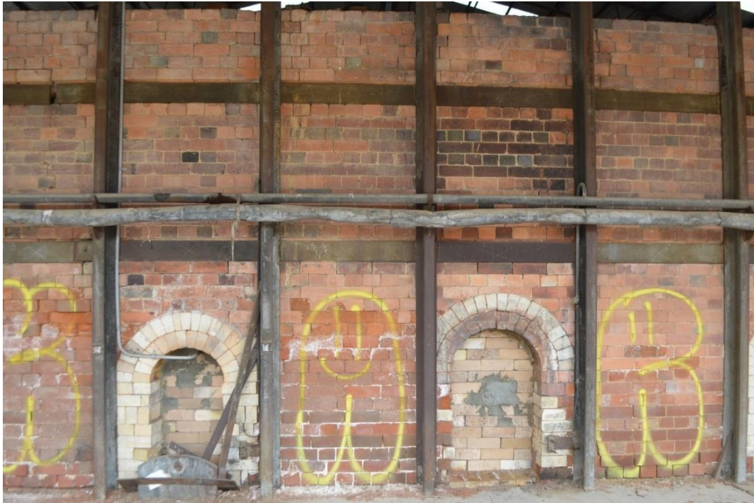
Figure 4.140 Two fireholes in the western side of the western Downdraught Kiln. The left firehole is connected to the subsurface flues, as indicated by the steel damper, whilst the right firehole leads directly to the internal kiln space.
