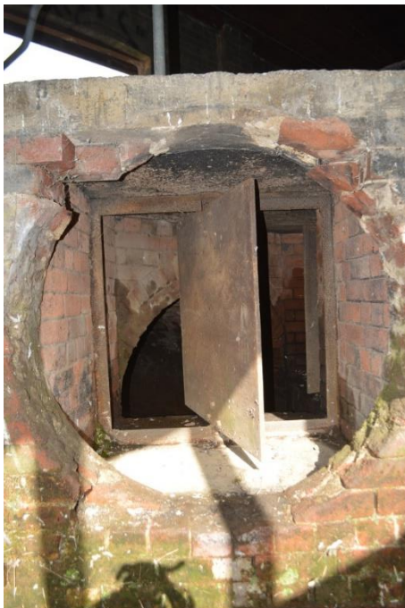
Figure 4.122 Entrance to the central tunnel via the fan house where the fan machinery has been removed.
