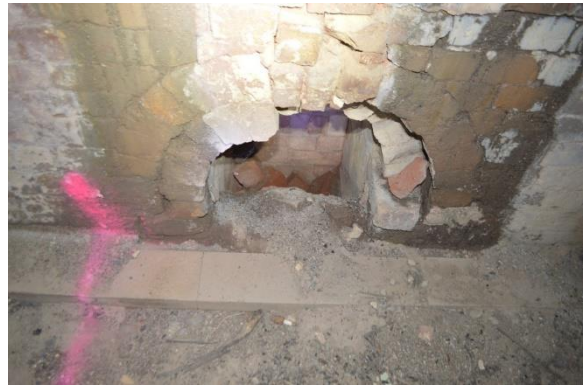
Figure 4.134 Brick rubble in the downwards shaft of a flue channel in the internal wall of the southern kiln chamber.
