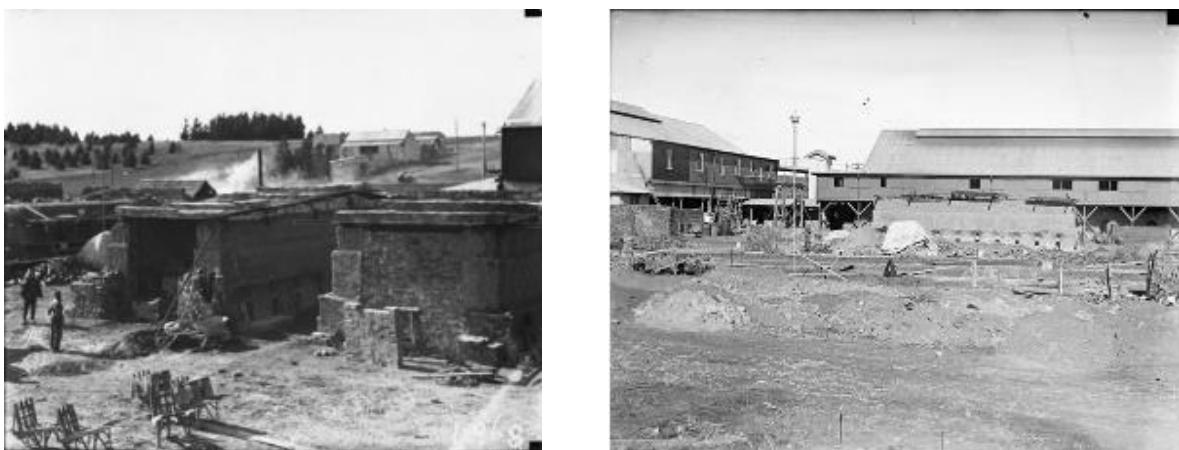
Figure 2.8 Scotch kilns (left) and a clamp kiln (right) were used to assist in making bricks for the Hardy Patent Kiln 1, c1926. (Sources: left, NAA, A3560 1968; right, NAA, A3560 1854)
