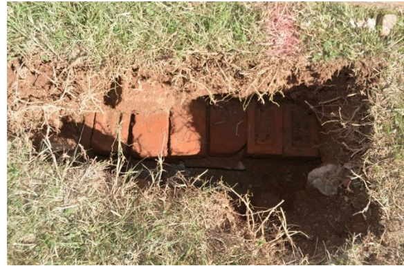
Figure 4.127 Part of a damaged remnant brick flue.
