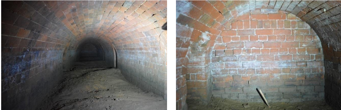
Figure 4.119 The central tunnel and rear wall, aspect southeast. Entrances to the smaller flue channels are visible in each wall of the tunnel.
