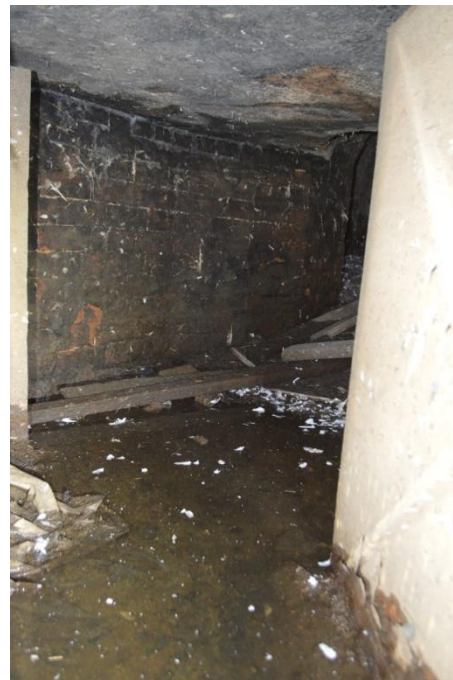
Figure 4.123 Split in the central tunnel where it funnels air through the fan machinery towards the chimney.
