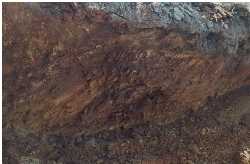
Photograph 7: Highly weathered, highly fractured siltstone with iron staining in fractures. TP16.
