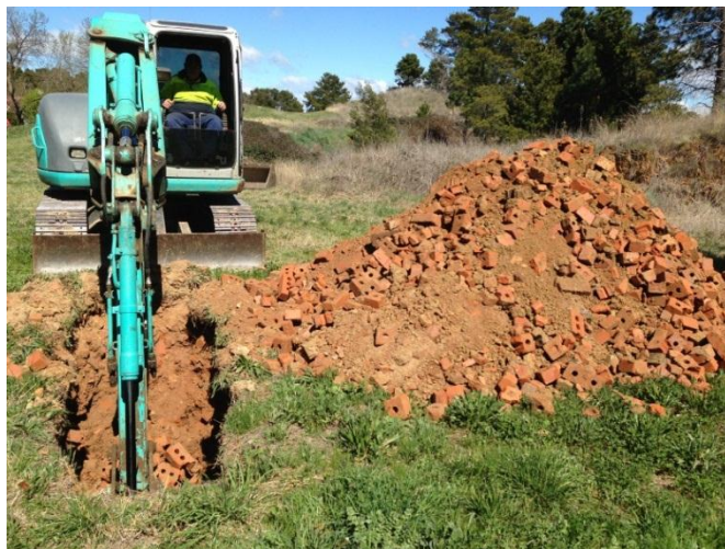
Photograph 10: Whole brick fill with clay encountered throughout the Quarry site. TP28.
